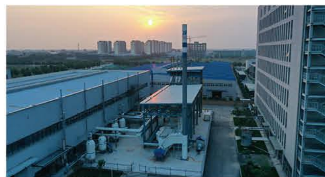
Supercritical Carbon Dioxide Cycle Power Generation Test Unit
