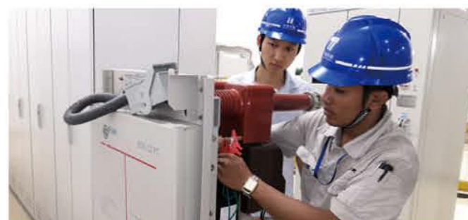
Cambodian Employees were Engaged in the Operation and Maintenance in the Station
