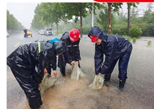
Anyang Thermal Power Plant Investigated the Pits of Road in the Area of Pipe Network
