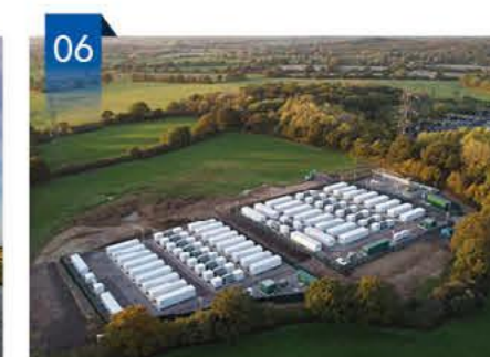
China Huaneng Group Hong Kong Limited: UK Minety Battery Storage Project Surrounded by Green Trees (by Guo Jingyu)
