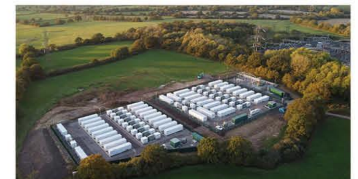
China Huaneng UK Minety Battery Storage Project
